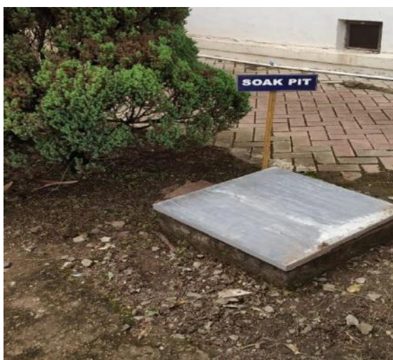
Figure 4: Soak pit for chemistry lab discharge
