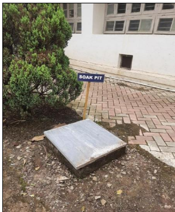
Soak pit for treatment of Gray water
