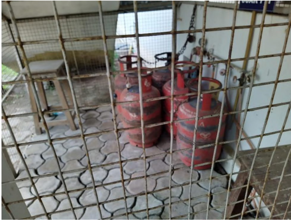
LPG cylinders placed outside the room and well protected with strong mesh.
